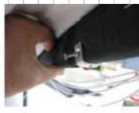
Fig.5 using small screw fasten blind rail to bracket. Take care not to snag the fabric on the screw.
